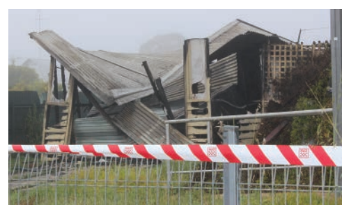
The fire in the Lilac Avenue shed was fuelled by a car that was also destroyed in the blaze. Picture: JENNY DENTON
